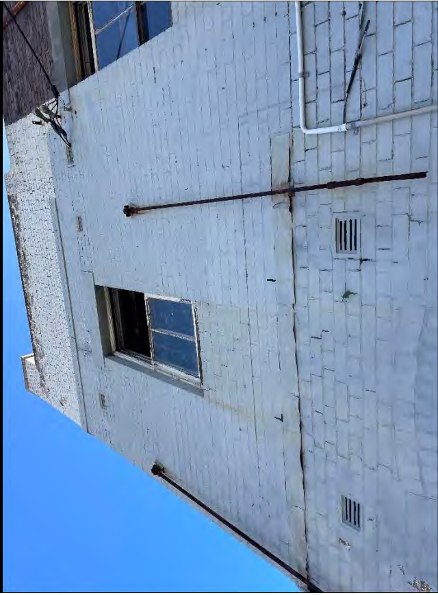
PHOTO 68: WEST BURWOOD, HISTORICALLY REPORTED AREA 1, UNOCCUPIED WAREHOUSE CONDITION
