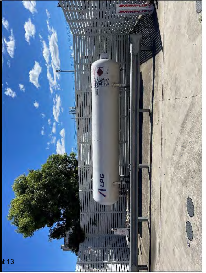
PHOTO 75: WEST BURWOOD, AREA 3, ABOVE GROUND LPG TANK IN WESTERN PORTION OF SERVICE STATION
