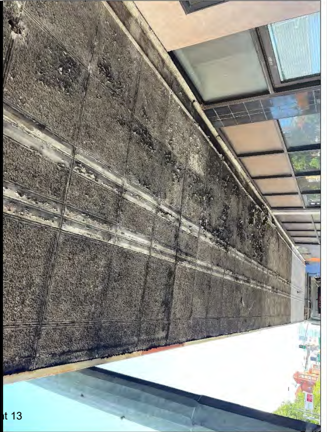
PHOTO 59: WEST BURWOOD, AREA 2, STOREFRONT STATE OF DISREPAIR OF STRUCTURE
