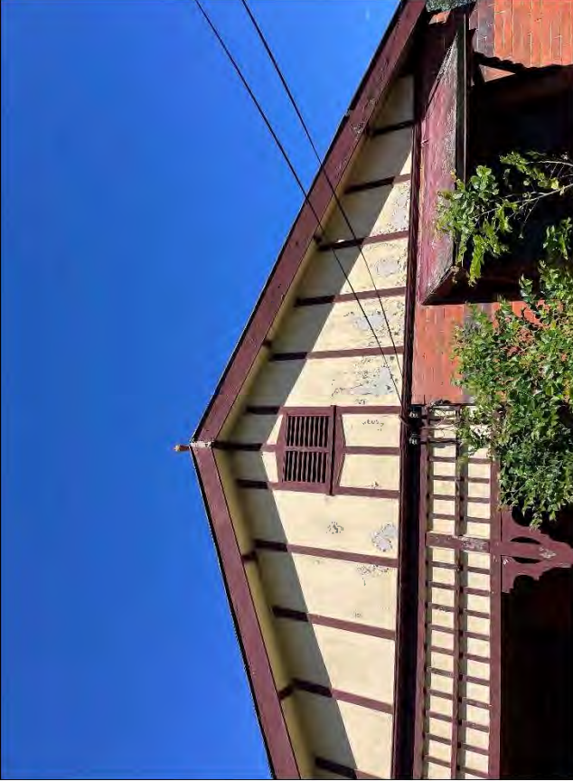
PHOTO 46: EAST BURWOOD, RESIDENTIAL AREA 10, RESIDENCE WITH PEELING PAINT
