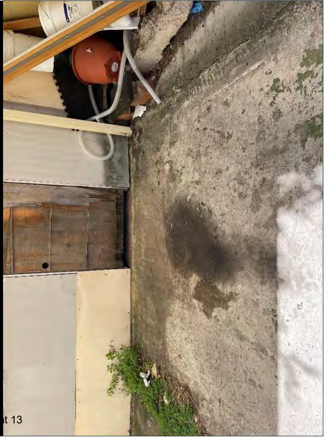
PHOTO 55: WEST BURWOOD, AREA 2, STAINING ON CONCRETE AT REAR OF DRY CLEANERS
